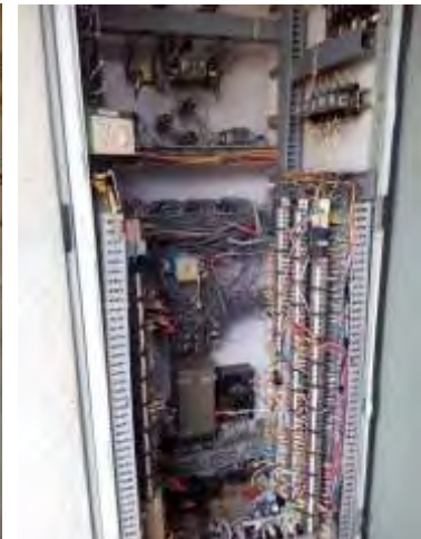
PT connections from KSEB's measurement PTs
